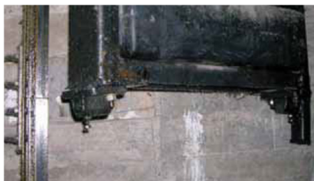
Figura 11 - Guide rotte o allentate Figure 11 - Guides broken or loose
